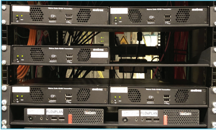
Matrox Extio 3 IP KVM extenders are integral to the centralization of assets at Fluxys.
